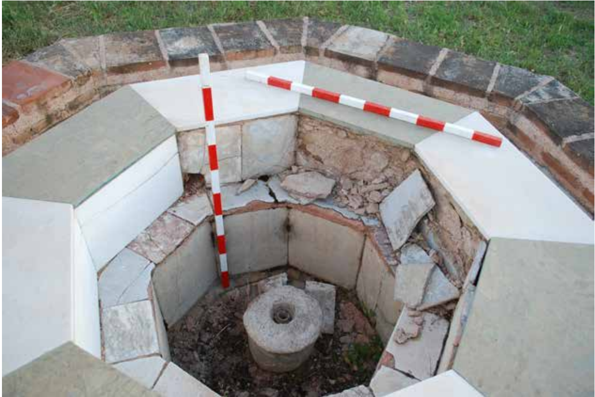
Fig. 59-62. Human hazards: examples of degradation due conservation activities made with inappropriate materials or lack of skills shortage and training
