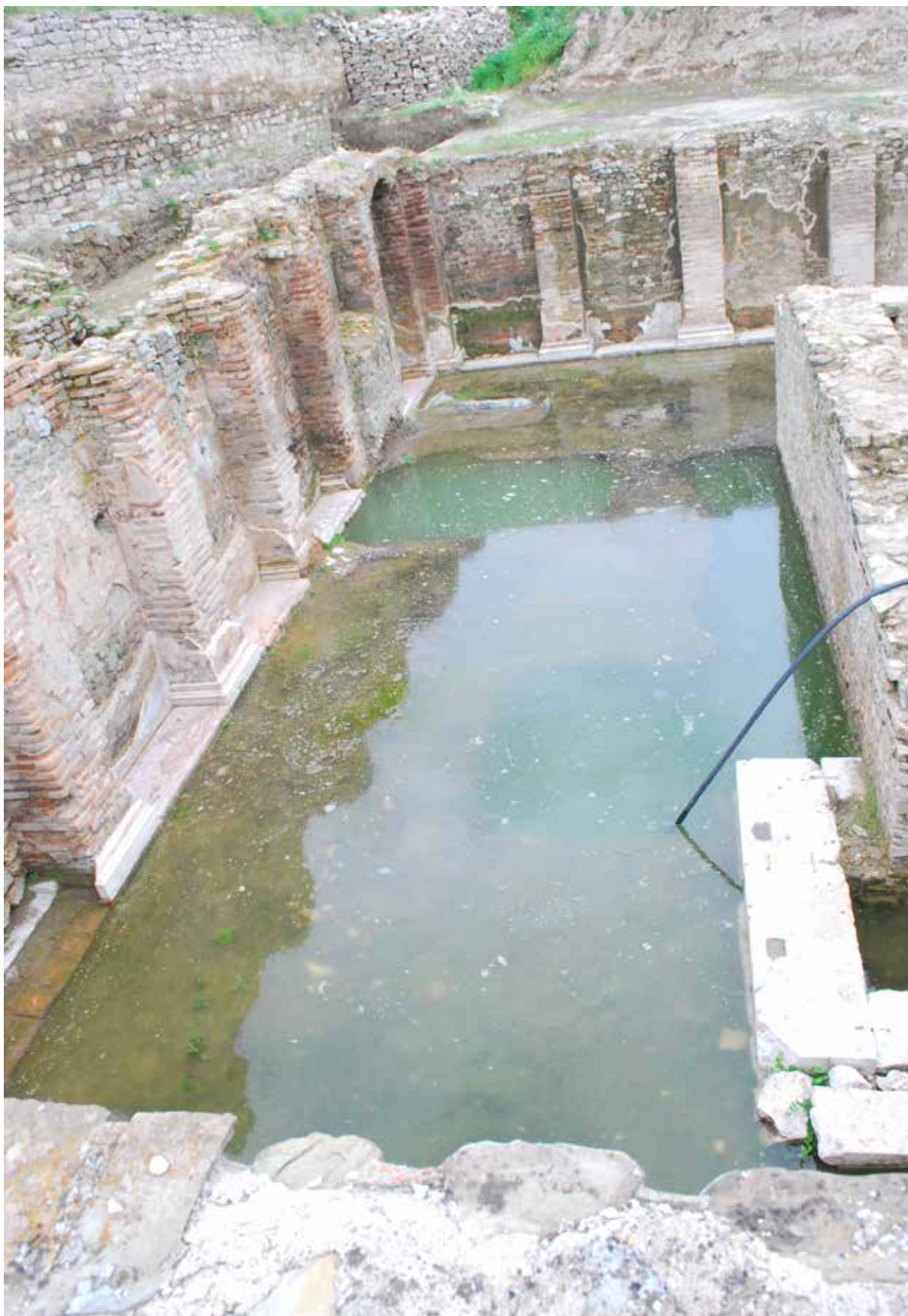
Fig. 40. Risk from flooding: rising of the subterranean waters and flooding in the Building with Arches, 2010
